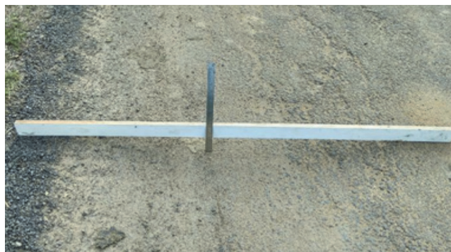
Figure 6. Rutting formed on the road surface in June 2017
